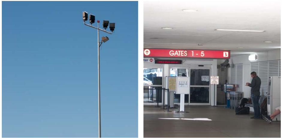
Noribachi's Interior and Exterior LED Lighting at Long Beach Airport
